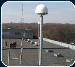
Base RTK Sart-Tilman
